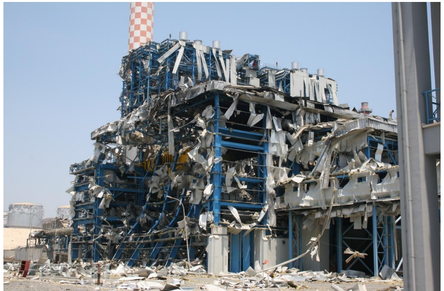
Photograph by employees of IDE Technologies Ltd. showing Vasilikos Power Station
